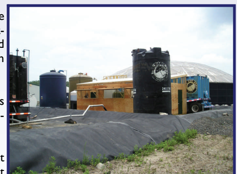
Pilot Study Campus: Permeate, Condensate and Concentrate Tanks, with RO Unit Housing.
