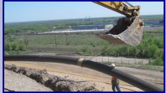
It can be a little tricky installing 500 lf of 12" pipe in a trench at one time
